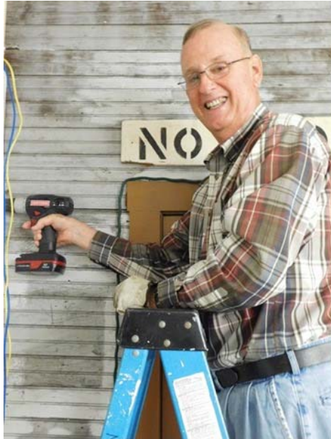
Society Member Phil Cross happily practicing his mastery of the drill while installing sheetrock in the new meeting room and museum expansion area.
